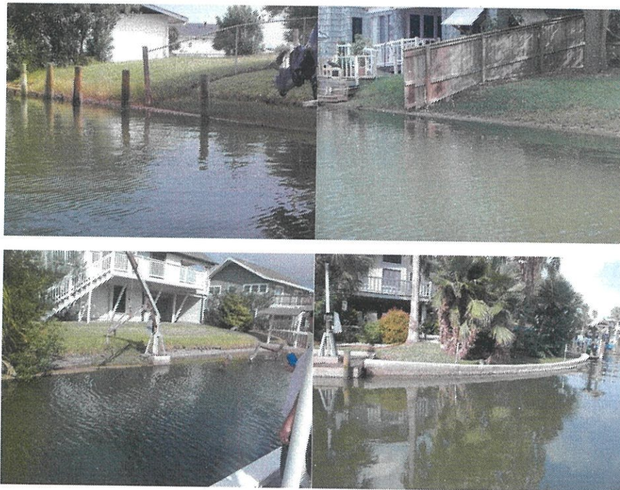
Figure 6: Examples of subsided bulkheads with limited freeboard
