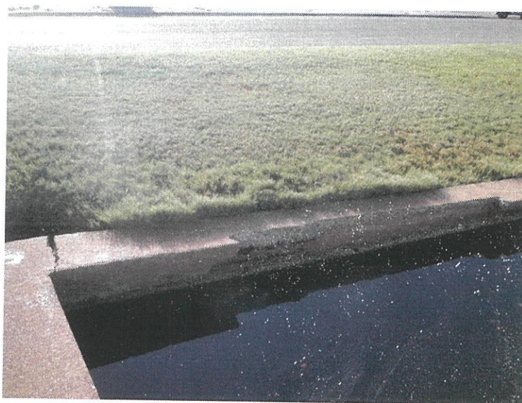
Figure 4: Deteriorating bulkhead cap
